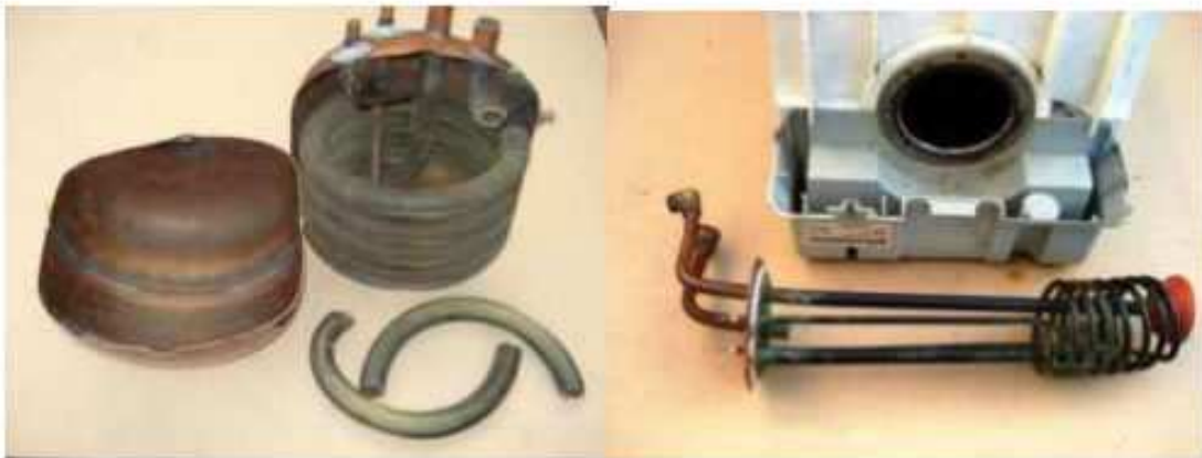
Figure 89 The insides of a domestic combi (left) and close-in (right) boiler. Both had been in operation for 12 years.
